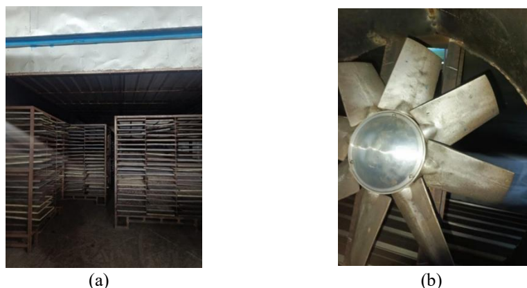
Figure 5. Experimental Briquette Drying Oven Used for CFD Validation (a) oven front view and (b) blower
